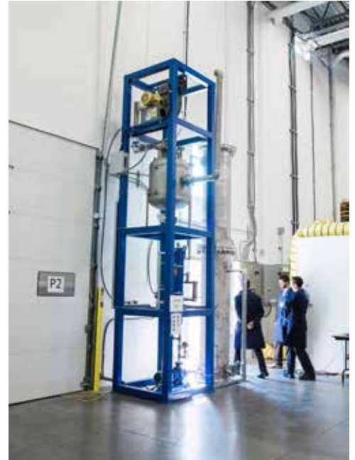
Flue gas conditioning system
