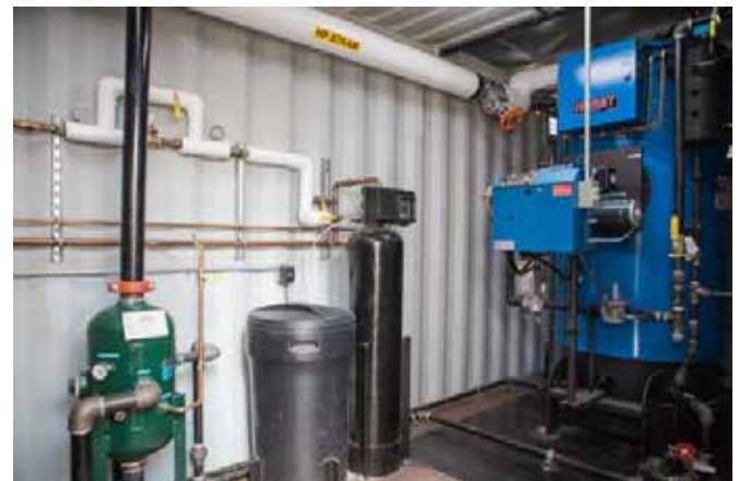
Industrial scale gas-fired boiler
